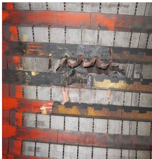
Typical core and winding damage resulting from a burned open bar in a slot
