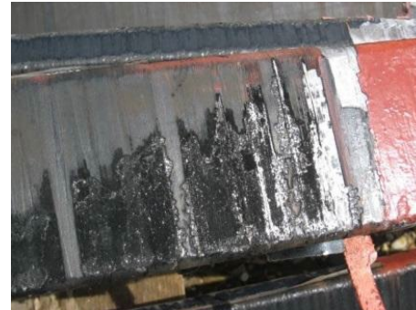
Side of a bar deeply damaged by vibration sparking
