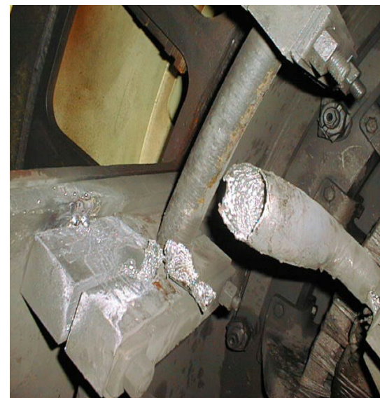
Typical winding damage resulting from broken stator winding conductor
