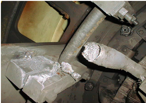
Burned away copper of a fractured connection ring
